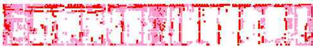
Figure 29: Combination of discriminant function results and initial segmentation. (individual images, Winnersh bridge, west face). Pink = classed as a defect / feature by discriminant; Red = reported by both initial segmentation methods.
