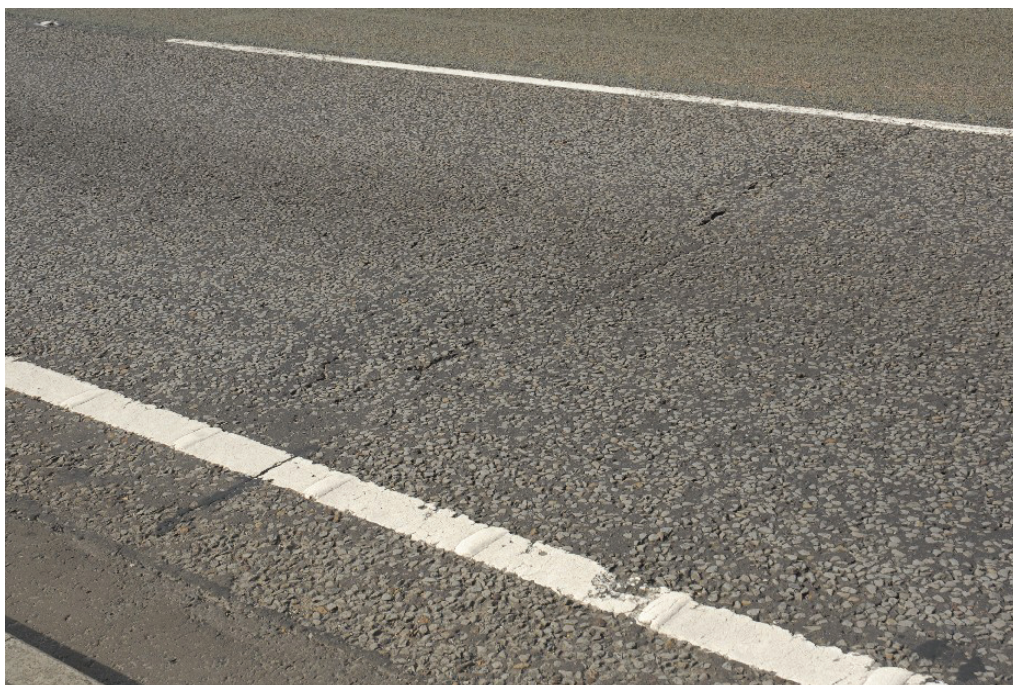
Figure 2.4: Irregularity in road surface at Site 2
