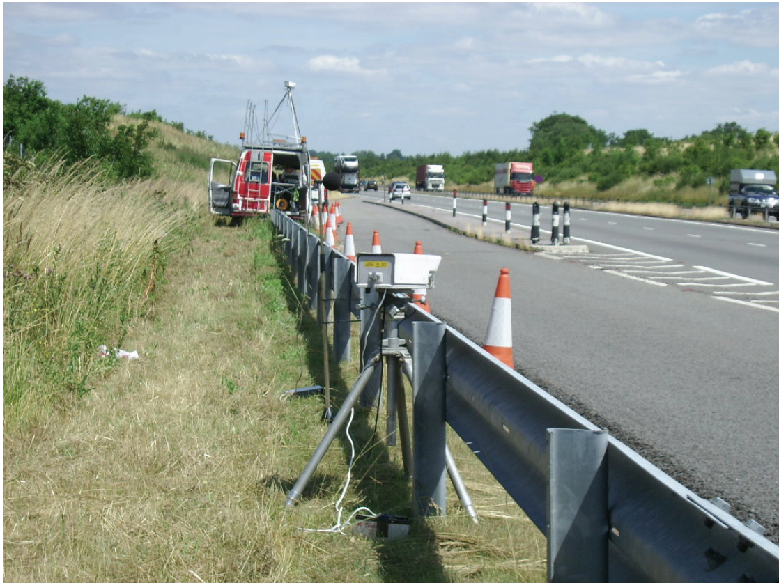
Figure 2.1: View of measurement set up at Site 1
