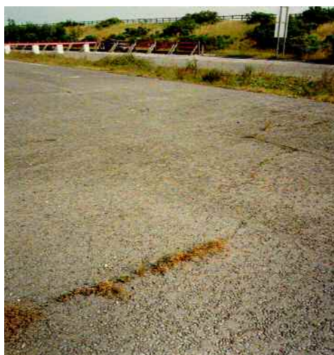
Fig 2. Reflection cracks in an untrafficked section of motorway
