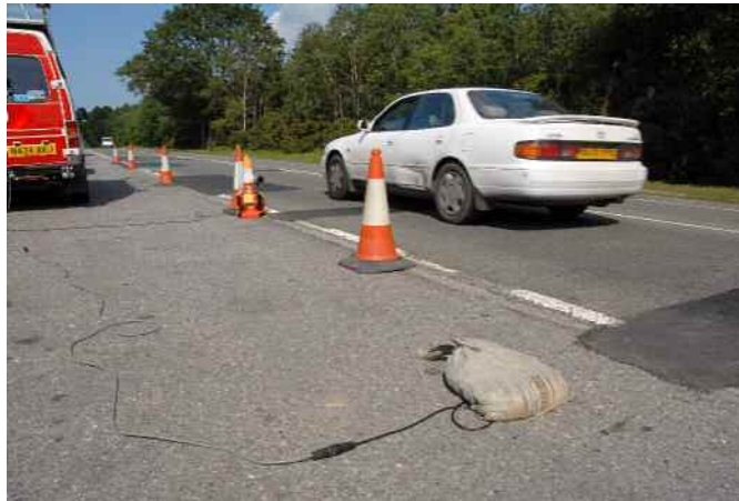
Figure 2.2: PPV transducer placed on the road surface (underneath a sandbag to ensure constant contact with the ground)
