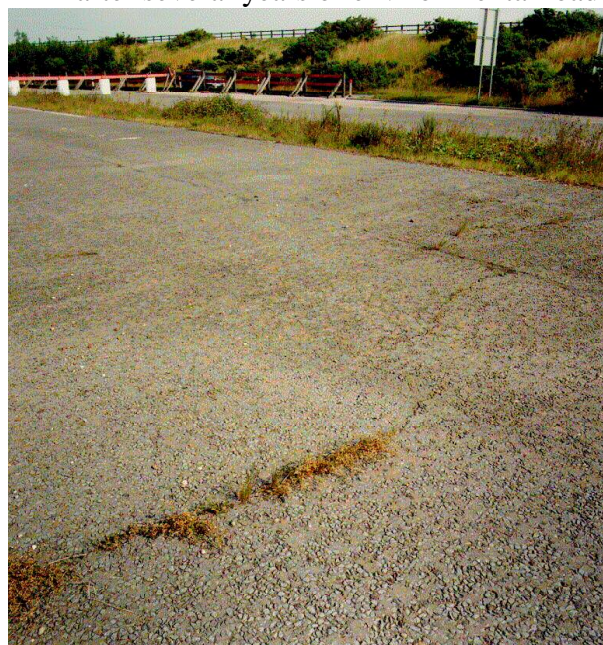
Figure 3. Reflection cracking in an untrafficked section of motorway.
