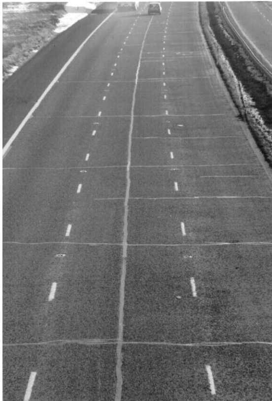
Figure 1. Reflection cracks in a typical UK composite motorway
