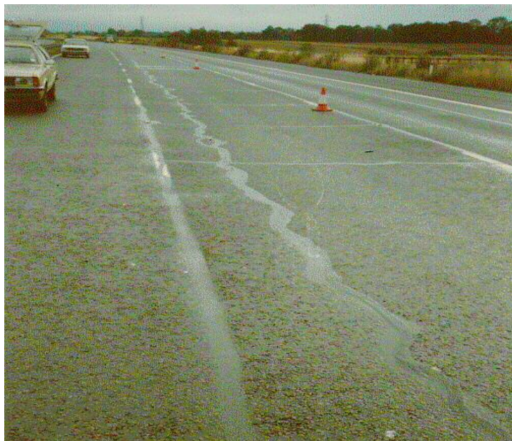
11 12 13 14 15 16 17 18 19 20 21 22 23 24 25 26 27 28 29 30 31 32 33 34 35 36 37 38 39 40 41 42 43 44 45 46 47 48 49 50 51 52 Figure 4. Reflection cracks in the centre lane of the M4 motorway
